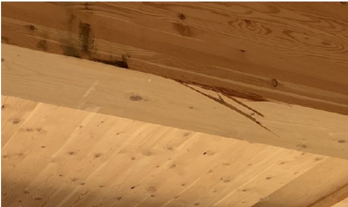
ABOVE Minor construction damage on the corner of a glulam beam
